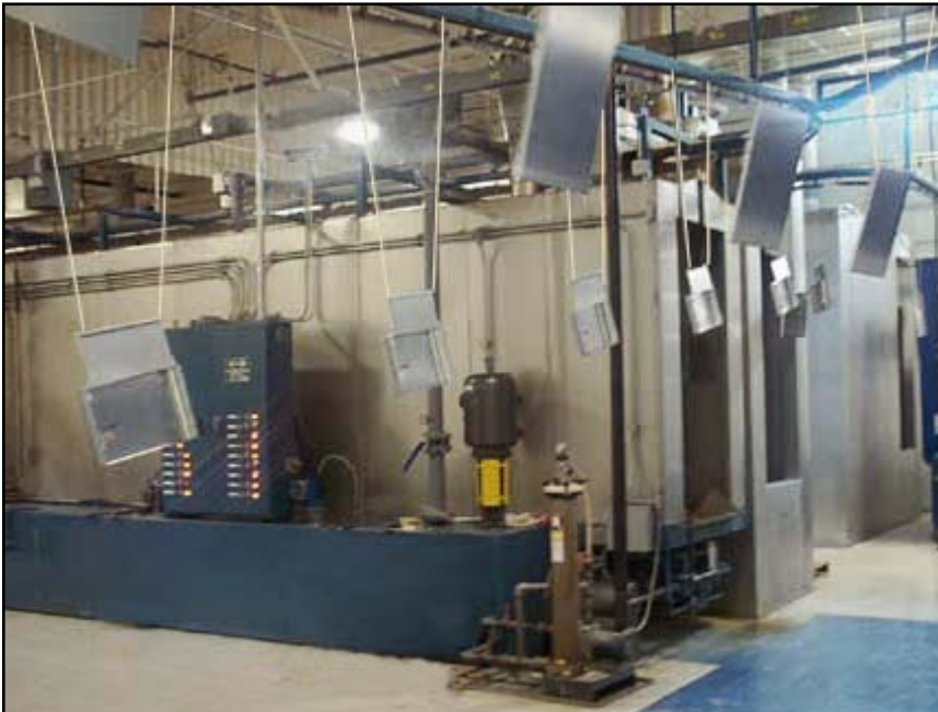
The automated wash system and dry-off oven.
